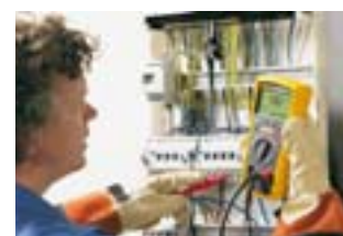
Insulation test at a distribution panel
